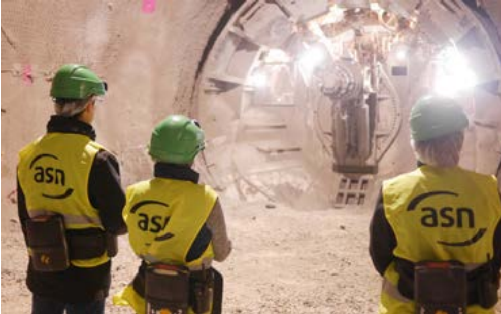
ASN visit during the excavation of the network of drifts in the Bure underground laboratory.
