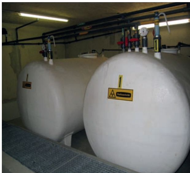
Decay management tanks for contaminated effluents from the nuclear medicine unit at the Beauvais hospital centre.
